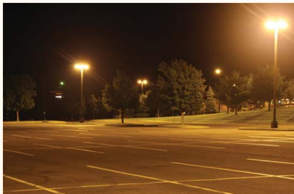
Outdoor lighting systems that provide full light output during periods of little or no occupancy waste energy.
