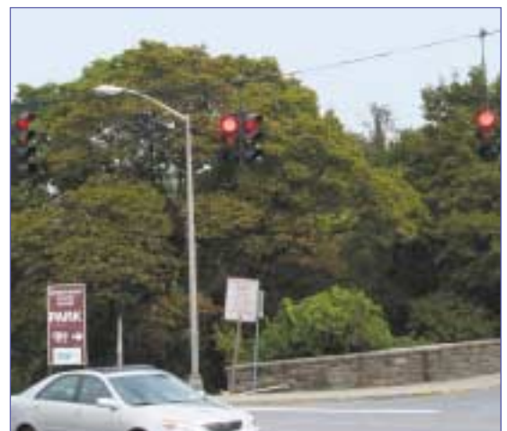
An installation of red LED signals in the Westchester County service area.
