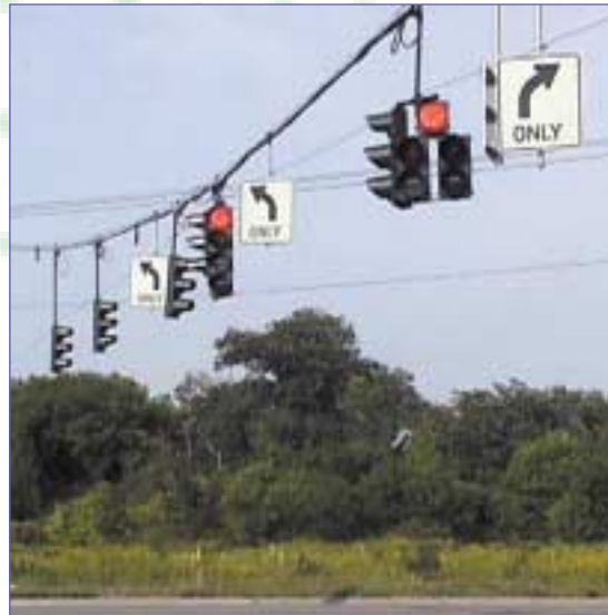
An installation of red LED signals in the NYSDOT service area.
