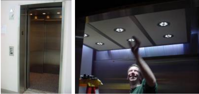
Figure 33. Photograph into the elevator cabin showing the existing incandescent lighting condition (left) and a photograph during the installation of the low-profile LED luminaires.
