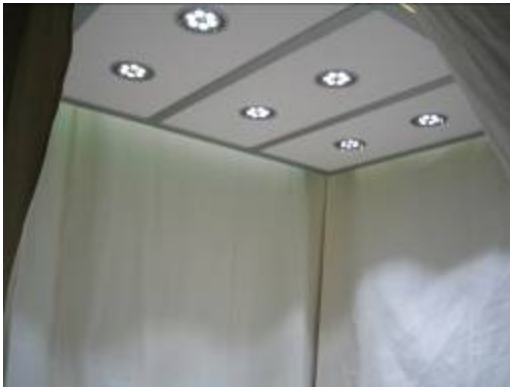
Figure 32. View from below the ceiling panel built for the field evaluation with the low-profile LED luminaires installed and functioning.
