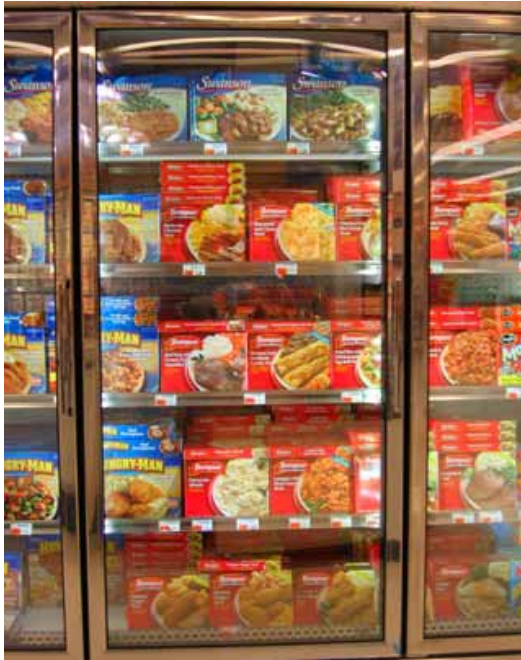
Figure 5. The LED freezer installed at Price Chopper.
