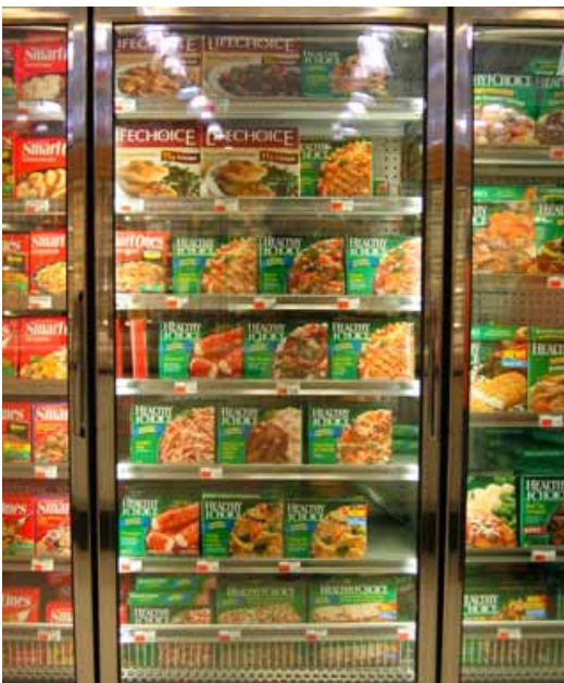
Figure 7. The fluorescent freezer installed at Price Chopper.
