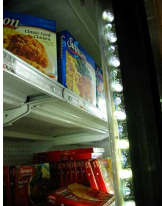
Figure 6. Close-up of the LED lighting system.
