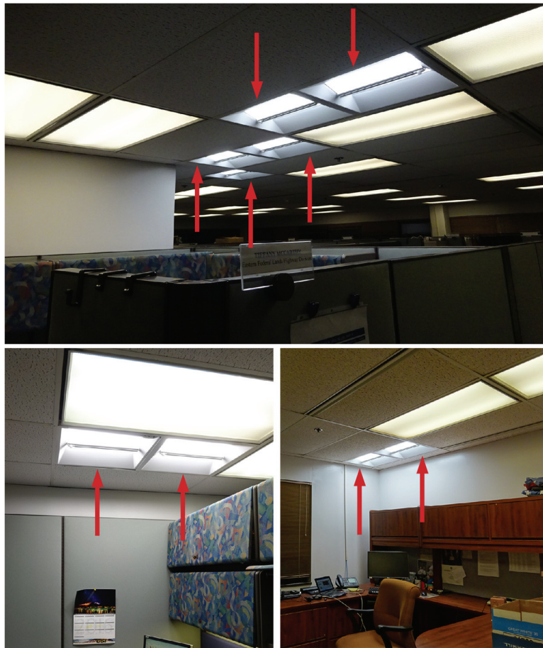
Fig. 4. Examples of the 2 \times 2 troffers (indicated by the arrows) used as lighting intervention at the FHWA site.
