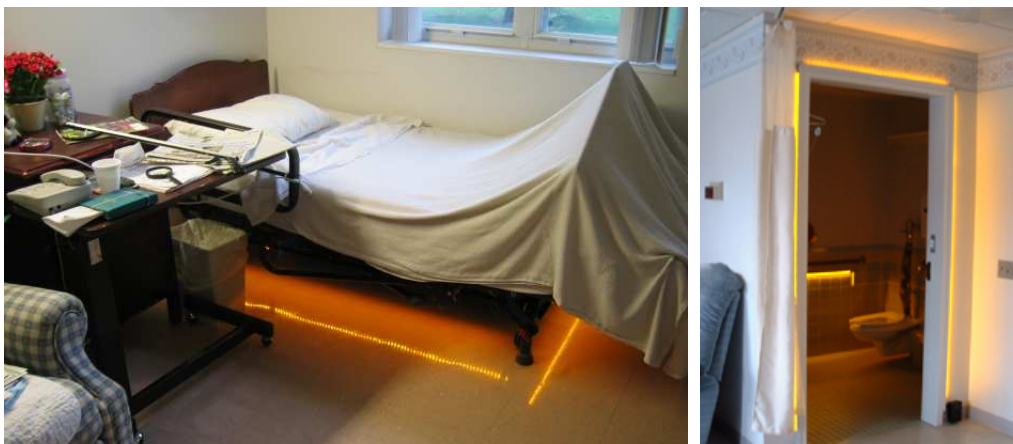
Figures 2a and 2b: Amber LEDs installed under bed (left) and around doorway (right). Note: photosensors were disconnected for the photos.
