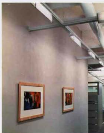
Wall washers highlighting perimeter wall
