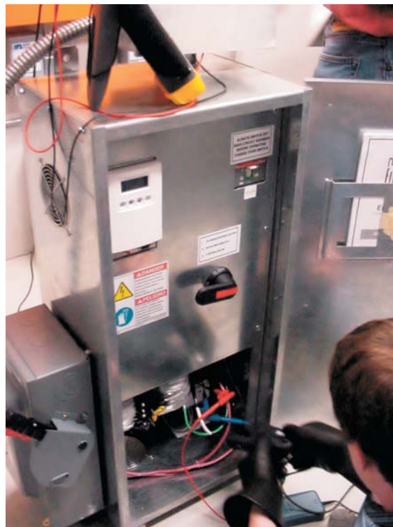
Figure 1. Electric City lighting circuit power reducer
