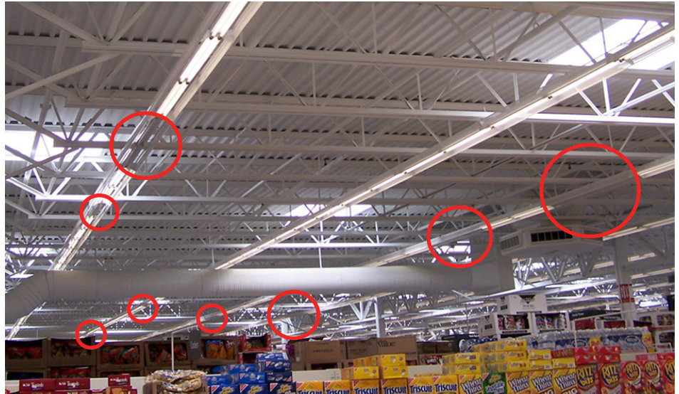
Some of the problems identified by Lighting Diagnostics investigators are circled above.
