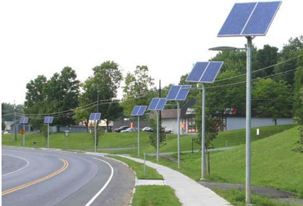
Figure 10. PV-powered luminaires used to illuminate a pathway
