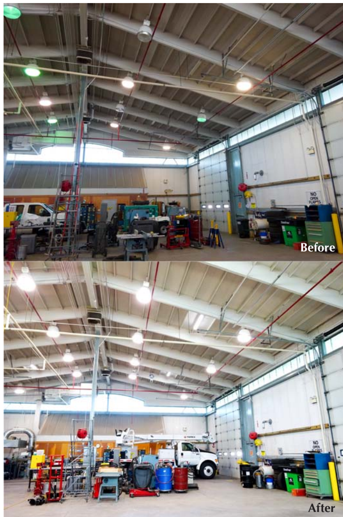
BPA Maintenance Facility before and after installation of LED replacement lamps
