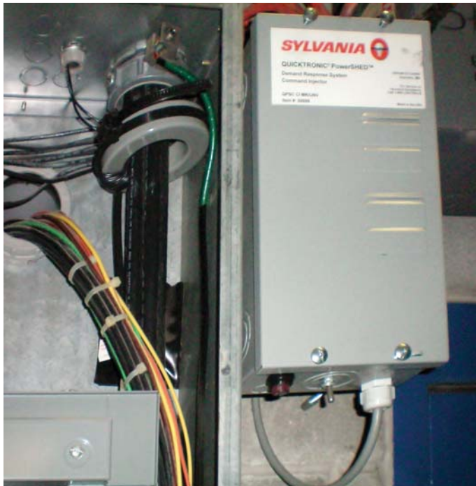
The signal injector uses a ferrite core (donut-shaped object around the electrical cabling) to introduce the load-shedding signal to the building's wiring at the electrical distribution panel.
