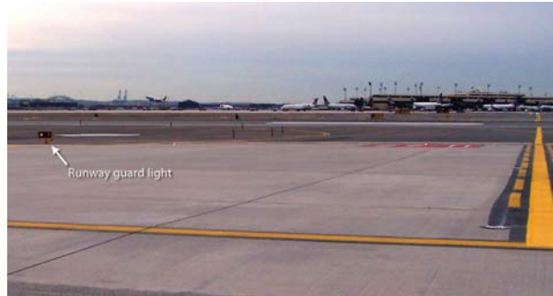
Runway guard lights on the airport tarmac.
