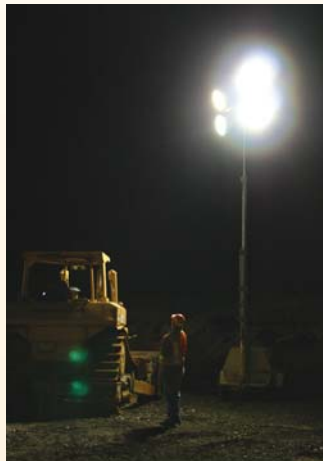
Trailer-mounted light towers introduce unwanted glare and sharp shadows, raising safety concerns in nighttime highway construction zones.
