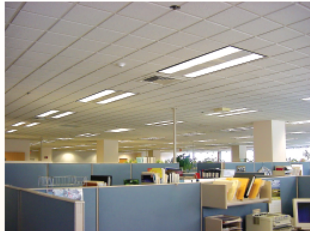
The LRC reduced ambient light levels by removing the center lamp from most luminaires in the open-office plan. To improve appearance, the dark center was covered with a panel similar in color to the ceiling, so that the luminaire looked like two single-lamp luminaires spaced close together.
