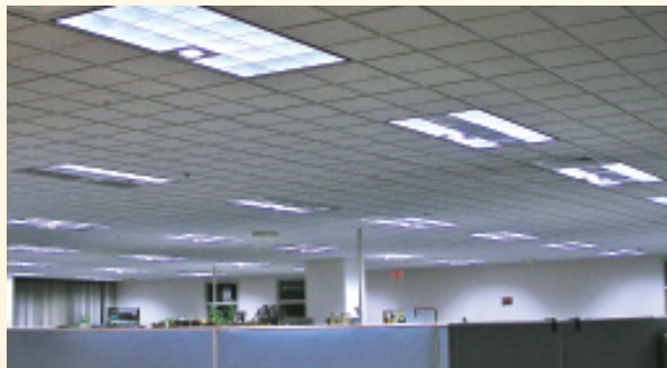
The LRC added sparkle elements to each luminaire seven months after lowering the ambient light levels. Pyramid-shaped diffused reflectors made of white, powder-coated aluminum created the "sparkle" effect.
