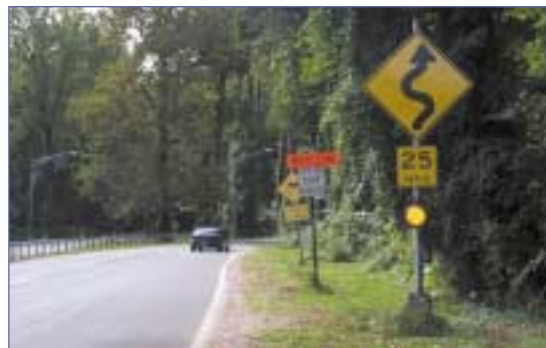
A yellow flasher LED installation in Westchester County.
