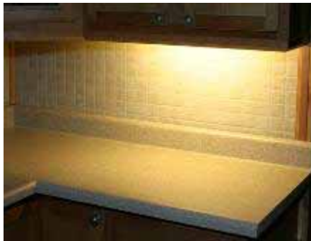
14 watt T5 linear fixture Average illuminance: 405 lux Minimum illuminance: 128 lux Meets recommendation for critical tasks? Yes Uniformity on counter: 3:1
