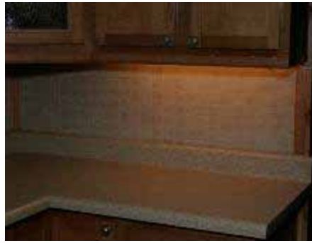
Low voltage halogen frosted festoon lamp light strip Average illuminance: 117 lux Minimum illuminance: 60 lux Meets recommendation for critical tasks?: No Uniformity on counter: 2:1
