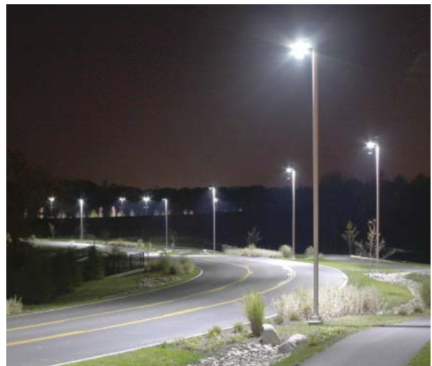
LED street lights along a suburban business park road
